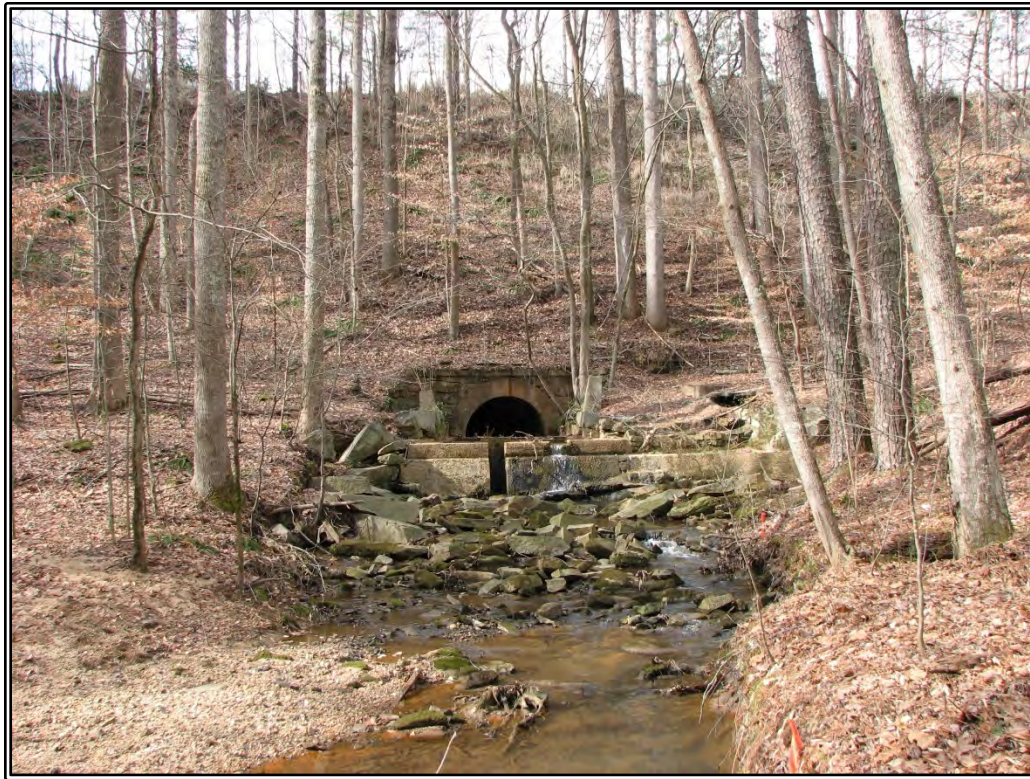
Figure 2. Photograph of Resource FK1270, pump station and the NC008 railroad berm, looking west from the Preferred Alternate Corridor.
